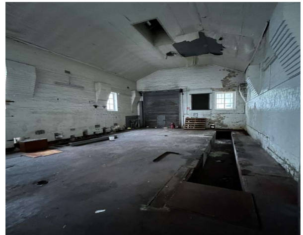
Figure 6 - Interior of the Substation facing northeast.
